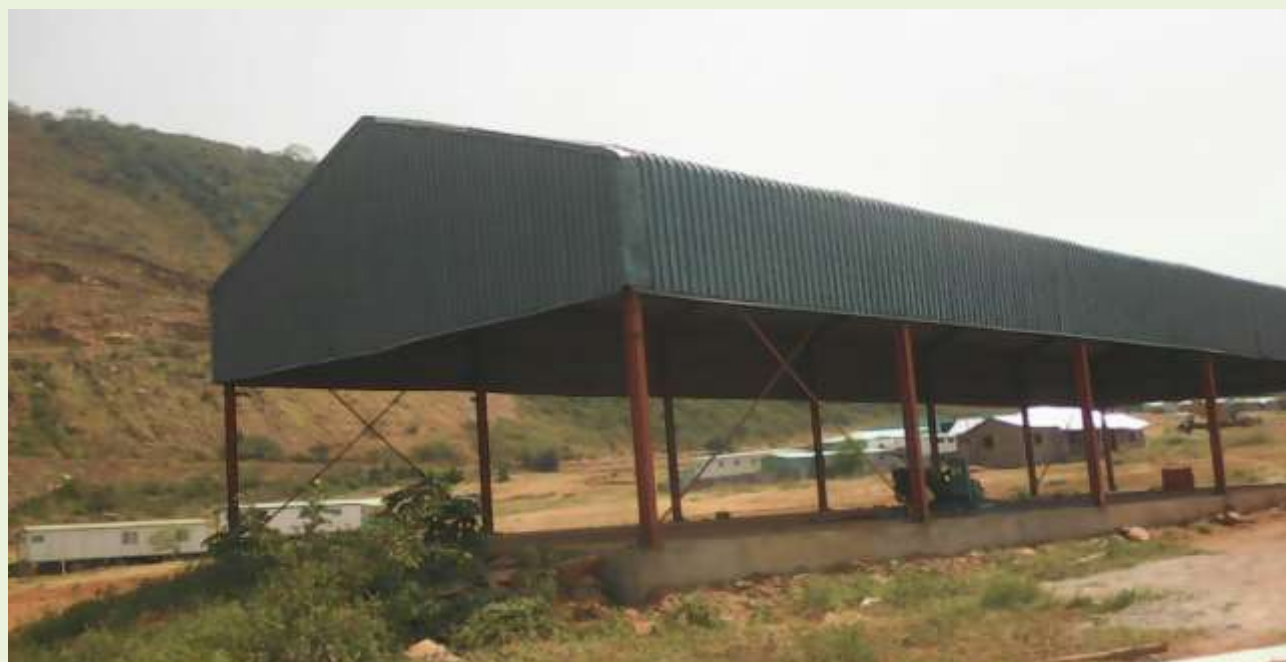
Fabrication and Erection of maintenance workshop at Hydro power station, Buliisa district, Uganda
